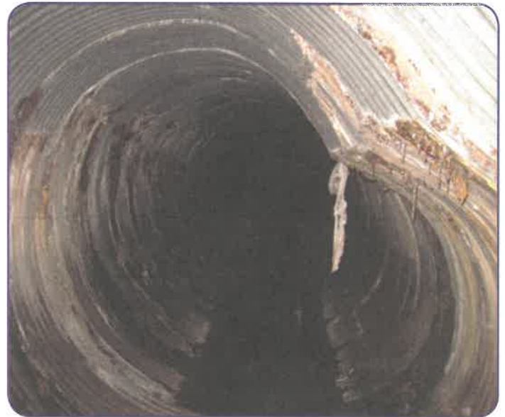
A buckled drainage pipe that could lead to another major sink hole. (2015 SDMP)
