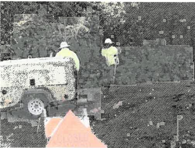
Worker using a shovel against asphalt at the T-junction of Via Farallon and La Cuesta, October 10, 1:30 PM
