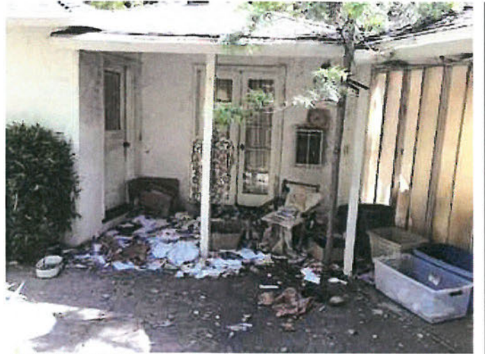
04/20/2022 Previously identified and noticed rubbish unmitigated, felled tree mitigated.
