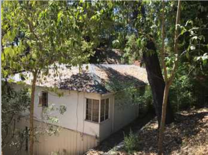
Final deadline is extended to 3/31/2022. Please clear leaves from the structure roof.
