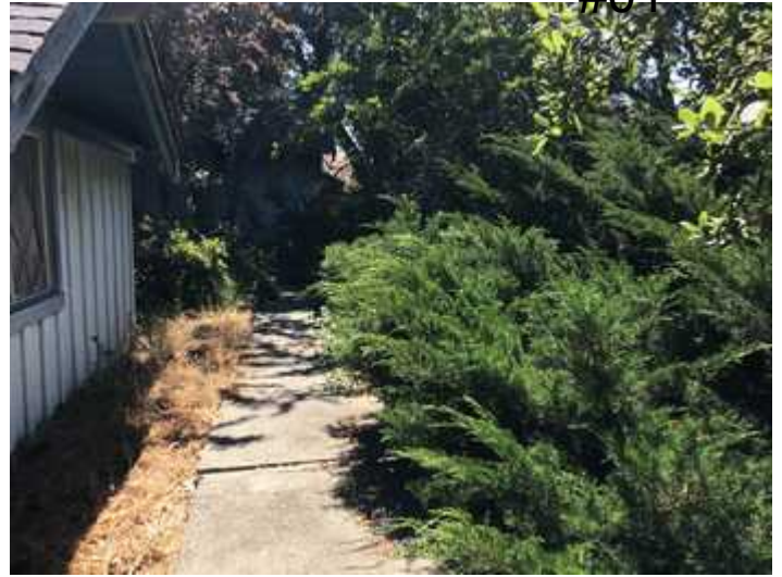
Cut back tree branches overhanging rooftop to provide 6 ft clearance.
